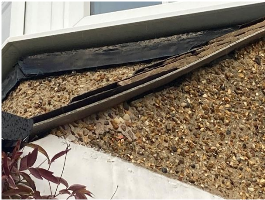
4 Deteriorated verge mortar to front bay roof covering
