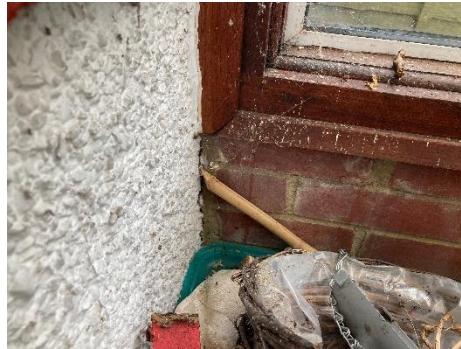
38 Cracking between structures
