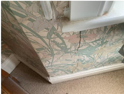
13 Differential movement to front bay structure
