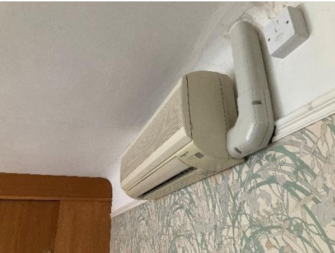
29 Air conditioning unit
