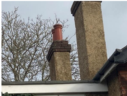
1 Weathered rear left hand chimney stack
