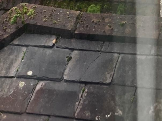
2 Cracked slates to single storey rear addition roof
