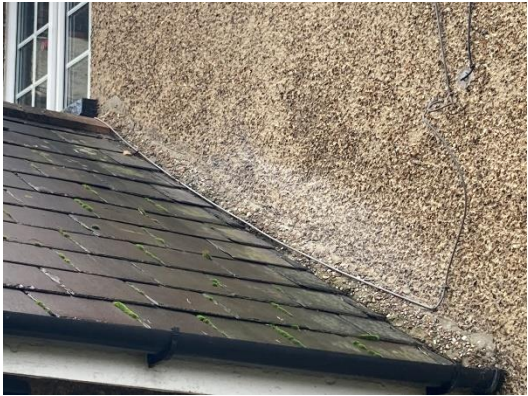
3 Mortar fillet to single storey rear addition roof
