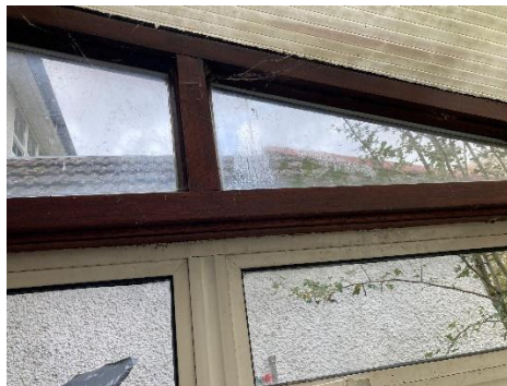
39 Failed double glazed seals
