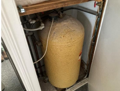
30 Hot water cylinder
