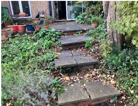
42 Loose uneven stones to patio/steps
