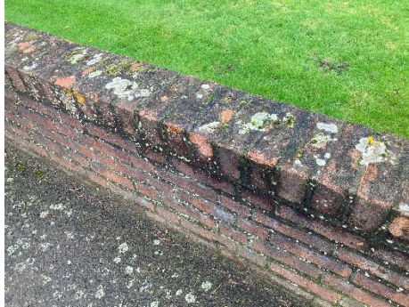
40 Weathered front boundary wall
