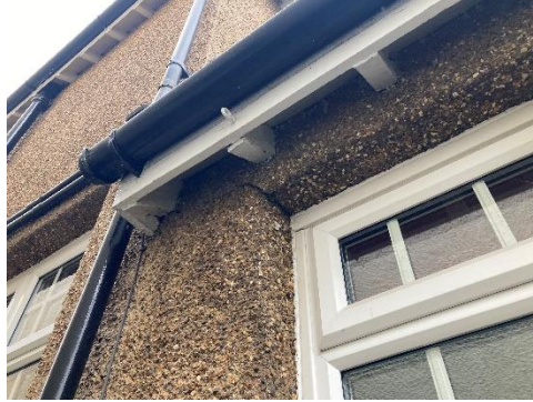
12 Cracking between main and single storey rear addition structures
