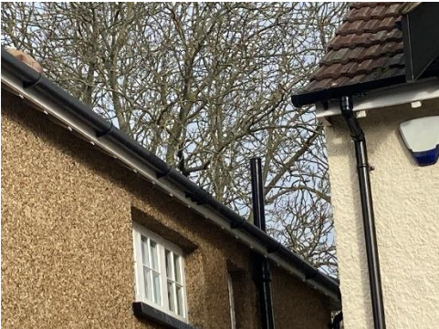
32 Uncapped soil pipe
