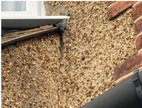
14 Differential movement evident to front bay structure
