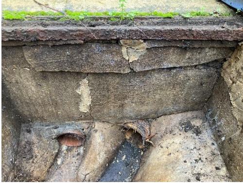
33 Cracked and damaged within drainage inspection chamber
