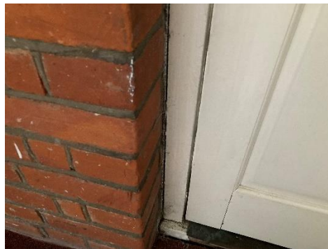
16 Gaps around door frame
