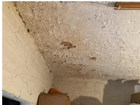
37 Past damage to ceiling
