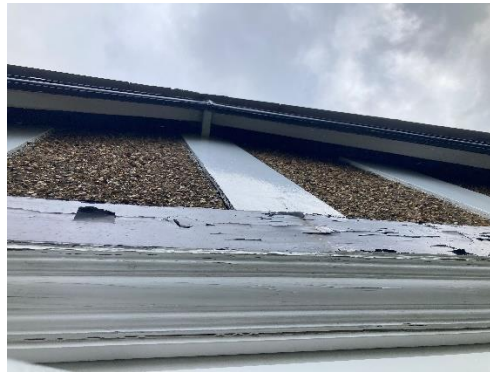
17 Weathered decorative timbers beginning to rot
