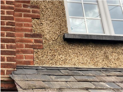
11 Cracking and distortion
